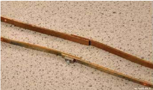
Fig. 6. Lap and bolted lap joints after short-circuit test.
